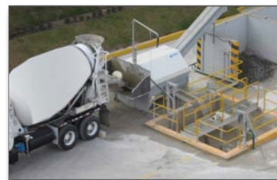
Figure 5. Ready mixed truck washing out into a reclaimer
